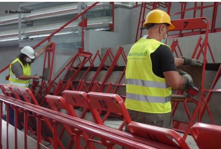
Social Urban Mining at Ferry-Dusika Stadium – removal of gallery seats for re-use (BauKarussell)
